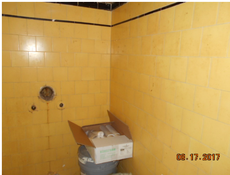
Lead-based ceramic tile, men's restroom storage (former shower).
