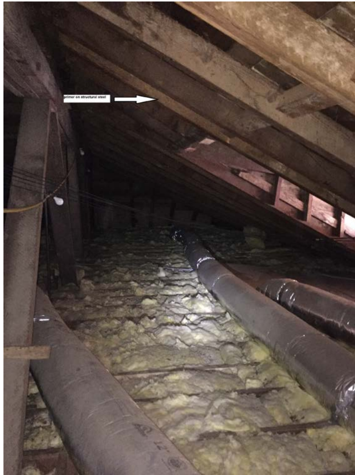
Primer on structural steel – assumed lead-based.
