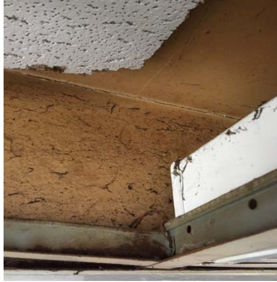
Yellow paint above north kitchen sub-ceiling. Lead-based.
