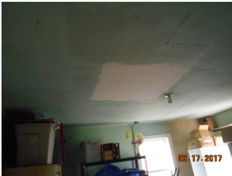
Green paint, ceilings, walls and baseboard. Lead-based.
