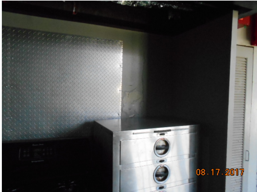
Gray paint on kitchen walls and cabinets– lead-based.
