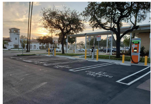
Costa Mesa EV Charging Station
