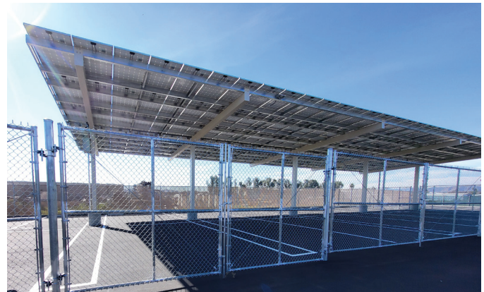
Parking Lot with Solar Riverside County Coroner Facility
